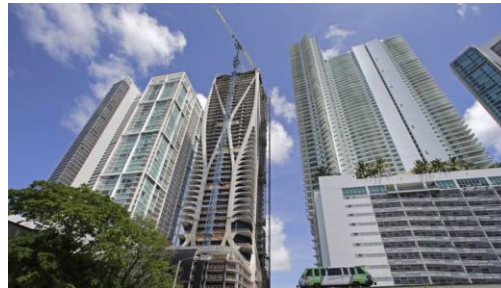
Penthouse Highrise building : Not down to earth
